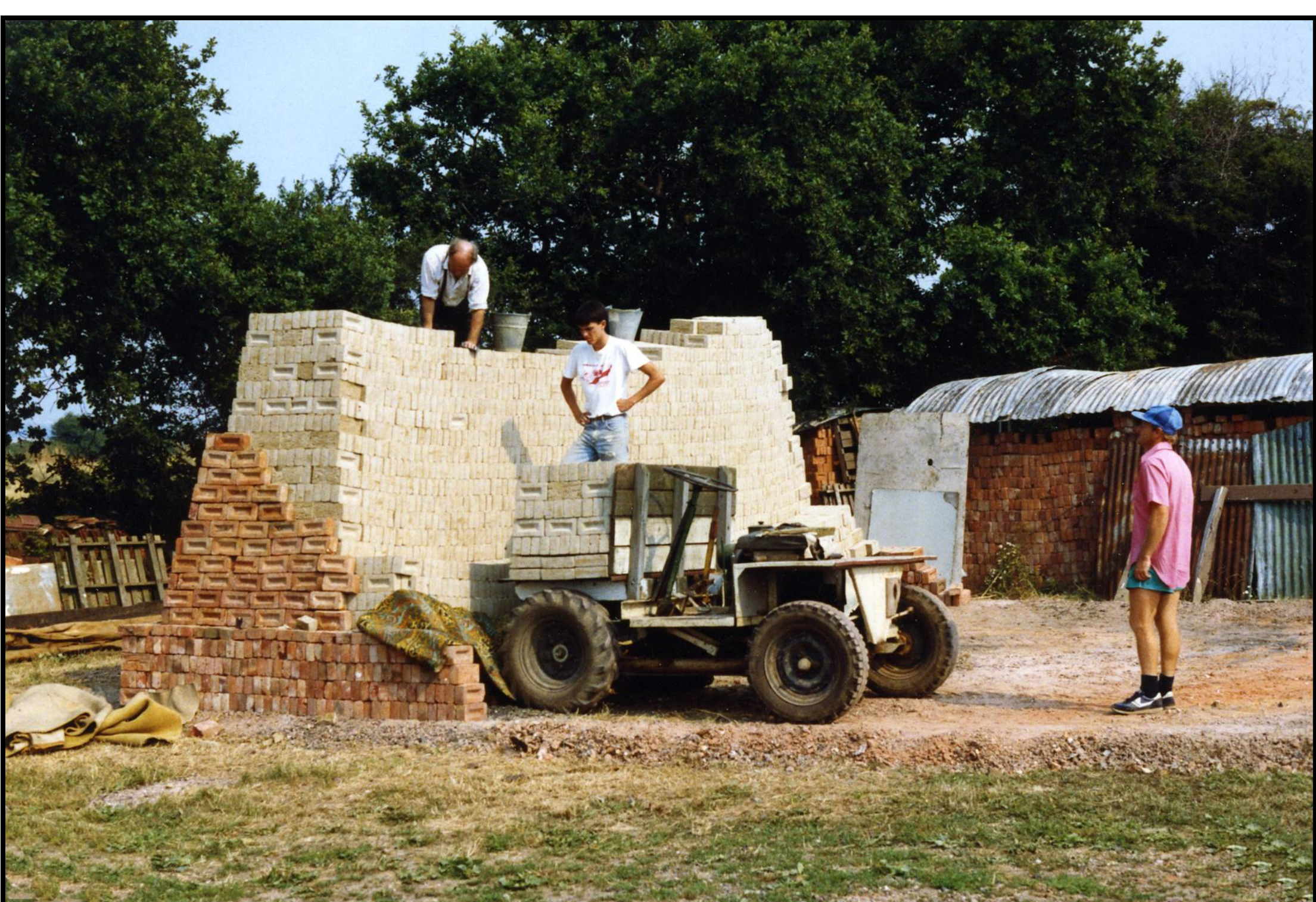
4.3. Bricks are carefully stacked with old bricks on the outside to help keep the heat in and to absorb the moisture. Fuel is built into the clamp as construction progresses.
